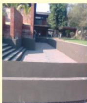
Swimming Pool Water Proofing System
